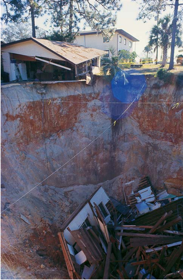
FIGURE 3 The remnants of a home engulfed as a large cover-collapse sinkhole developed over several hours, Keystone Heights, Florida (east of Gainesville). The occupants were able to evacuate safely, although their Christmas tree and presents were lost. The surficial sediment is clayey sand, which spans the upward eroding subsurface void allowing it to grow to a significant size before it collapsed. The limestone at this location is approximately 100 feet below the land surface. (Photograph courtesy of Barry F. Beck.)
